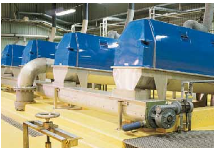
Roto-Sieve drum screens, model RS-51, installed at Kullavik treatment works in Kungsbacka.
